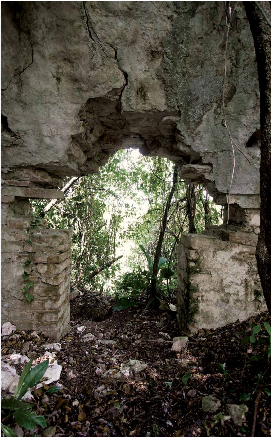
Figure 45. Budsilha Structure 1, looking west through the doorway in the median wall between the eastern and western galleries, 2010. Photo: Andrew Scherer.
