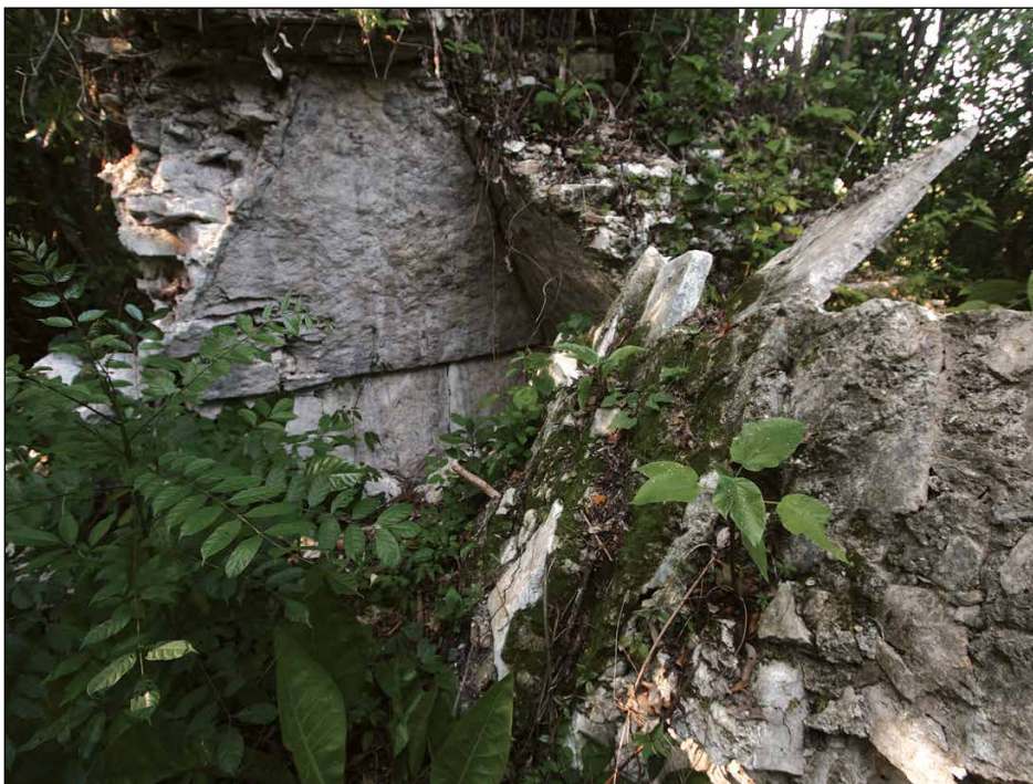
Figure 44. Budsilha Structure 1, collapsed center wall, 2011. A portion of intact vault in Figure 42 is lying in the foreground of this photograph. Photo: Andrew Scherer.
